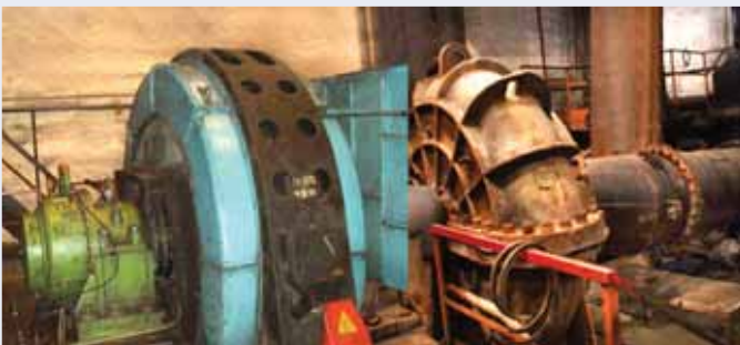
Iron Ore Mud Pumps at 6000V / 500A (Synchronous Motors)
