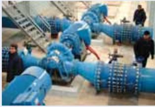
Three City Municipality Fresh Water Pumps 3300V / 300A
