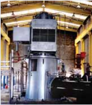
Four City Municipality Water Pumps at 4160V / 400A elevating Fresh water to 1800 Meters
