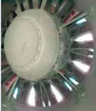
Four Air Supply Fans in a Gold-Mine 6600V / 300A
