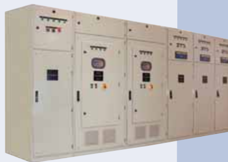
Single supply with two redundant soft-starters, where any starter can start any of the three fire extinguishing pumps 3.3KV, 110A
