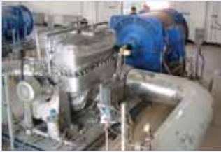
Liquid Gas Booster Compressor 6600V / 600A
