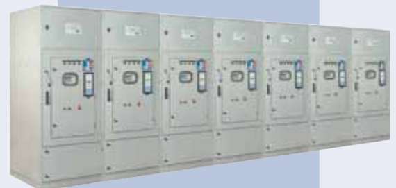
Medium voltage MCC lineup with load make fault break switch, fuses and a protection relay.
